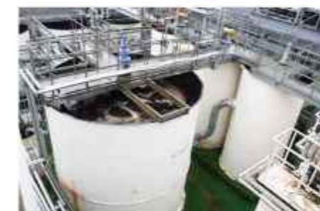
Wastewater recovery system
