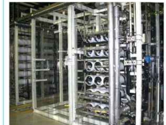
Recovery of Phosphoric Acid (H 3 PO 4 ) System
