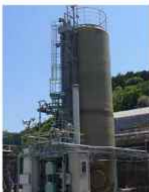
Anaerobic wastewater treatment system using a carrier
