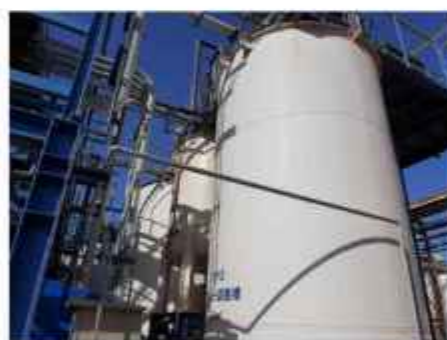
Wastewater treatment facilities
