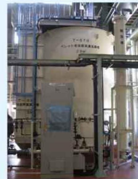
Pellet-forming high-speed coagulation and sedimentation device
