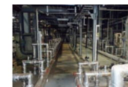
Wastewater treatment facilities
