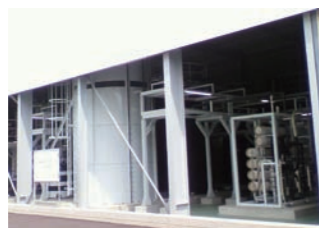
Wastewater recovery system
