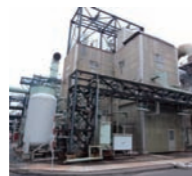
Flue-gas desulfurization equipment
