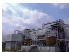
Wastewater treatment system
