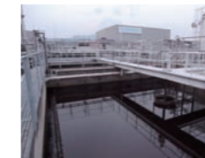
Coagulation sedimentation equipment
