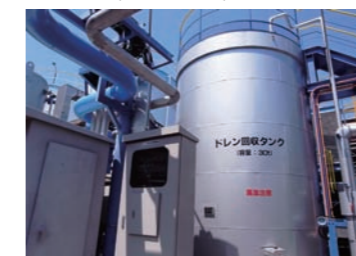
Steam condensate recovery system
