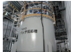
Waste alkali liquid treatment system
